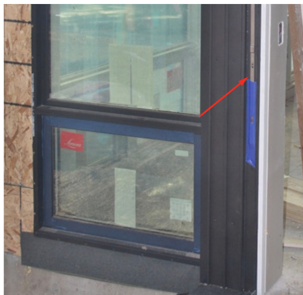
Interior track with spike plate
