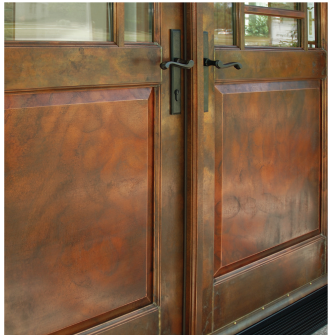
Raised exterior panel.
