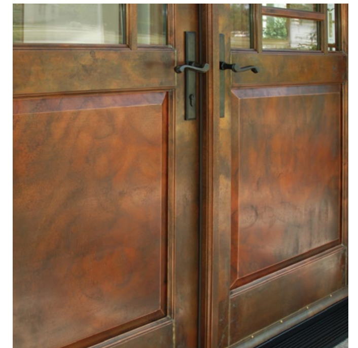
Raised exterior panel.
